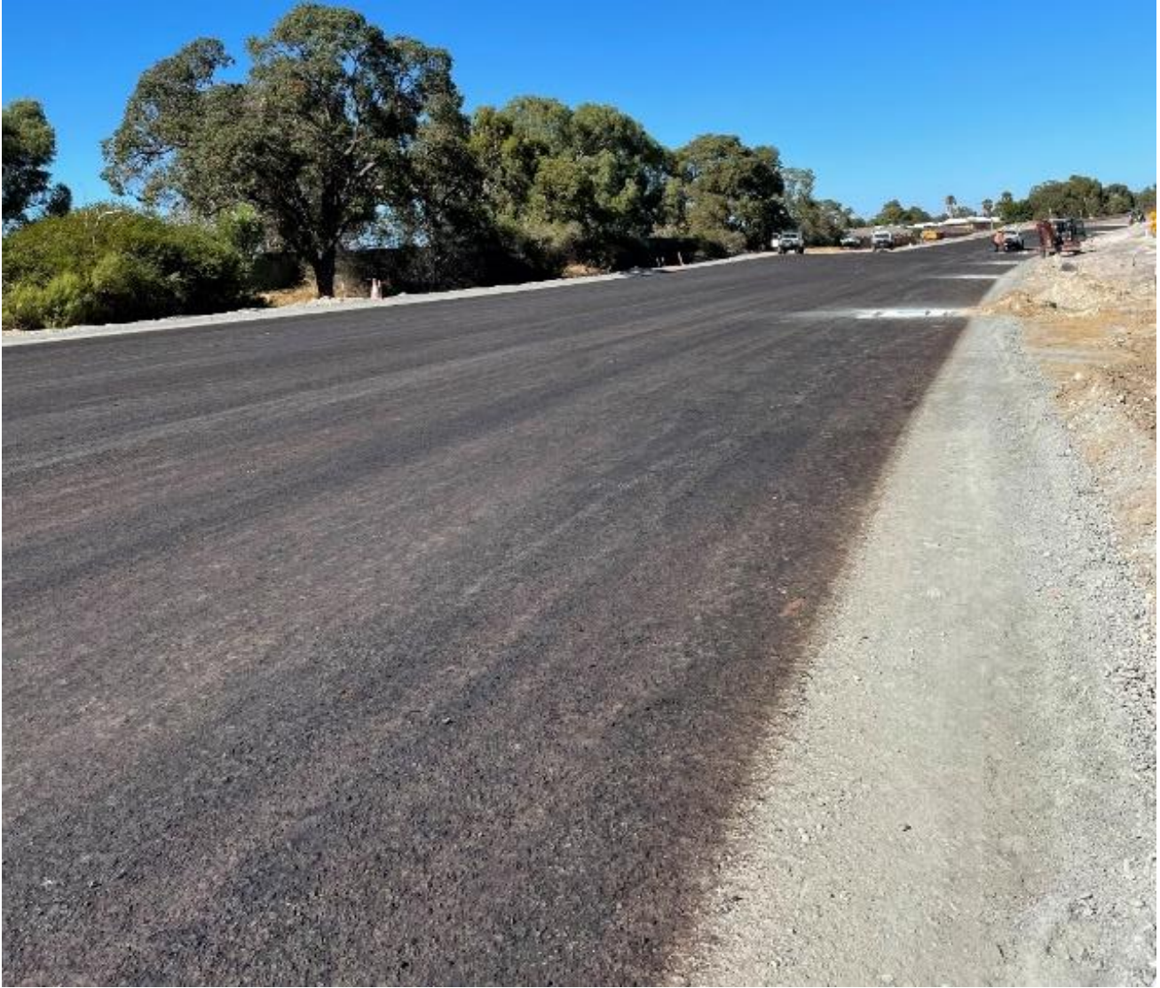
Figure 7 Pavement Construction – Prime application Leach Highway Southbound, facing South, on crushed rock granular basecourse. This is the first step in the construction of the bituminous surfacing layer
